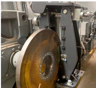
The brakes for elevation, the mounted winch and hoist were all replaced.
