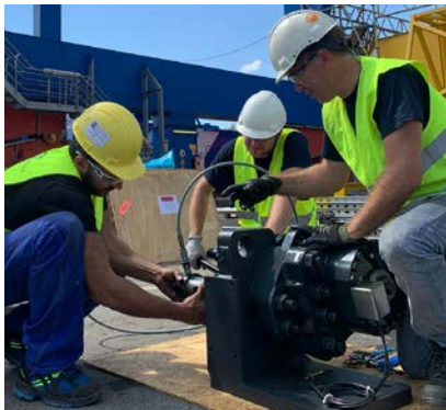
Stromag's service team commissioning the intelligent crane monitoring system utilizing Industrial Internet of Things (IIoT) technology at the world's largest inland port.
