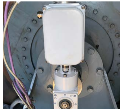
Geared cam limit switches matched with encoders were installed, which provided data on position, speed, overspeed and possible faults.
