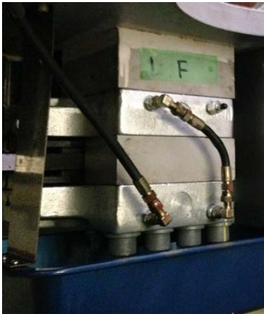
Fig 1: Assembly inside Nacelle before retrofit.
