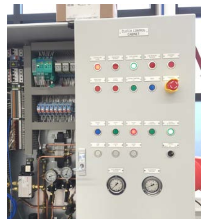
Typical Wichita clutch control cabinet and panel
