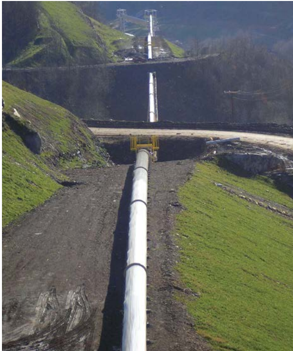
400hp coal conveyor at Browns Creek Complex – Rupert, West Virginia, drops 468 ft. over a length of 1230m.
