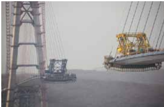
The central span of the bridge is made up of 103 panels, each 12m long, 26m wide, and weighing 300 tons.
