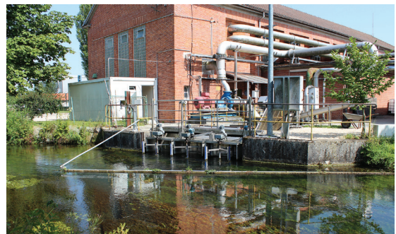
In river water extraction applications, the ability of the motor system to cope with demanding environmental conditions is of paramount importance.
