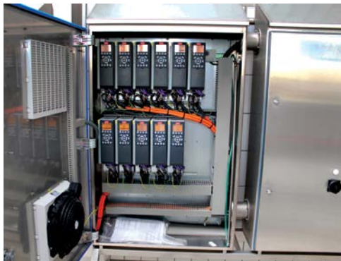
Variable speed drives ensure conveyor speeds are matched precisely.
