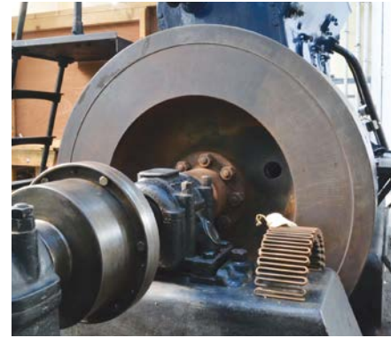
The Bibby coupling was installed to transmit torque while protecting the critical engine and gearbox from potential damage due to vibration and torsional shock caused by the long pump driveshaft.
