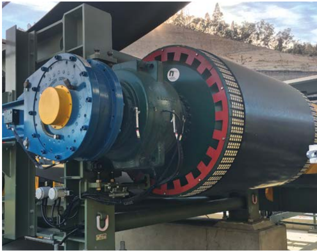
Dual RDBR 300 models with 70 kNm torque per unit are installed on the 1800 mm (5.9 ft.) wide, 3,050 m (1.9 mile) long drift conveyor at the Moolarben mine that transports coal from the longwall system underground to the surface. The inclined conveyor features an 80 m (262 ft.) lift and has a capacity of 4,500 tph.
