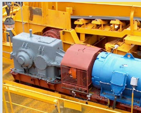
Spring-applied, hydraulically-released BSFI 320 brakes act on a 0.8 m (2.6 ft.) diameter disc mounted between the electric drive motor and the gearbox on the high-speed side of the drive. The brake system can provide 60 kNm of torque max. and allow for controlled braking up to 50-seconds in case of a power failure.
