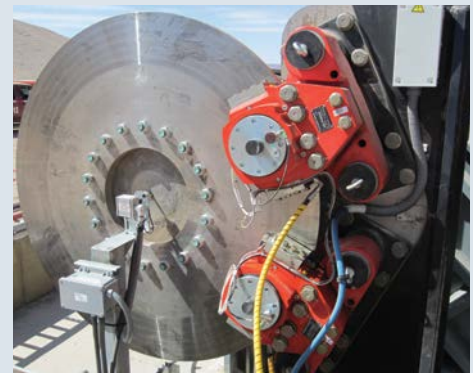
Spring-applied, hydraulically-released BSFH 520 brakes act on a 1.6 m (5.2 ft.) diameter disc mounted on the low-speed side of the drive shaft. The brake system provides up to 134,354 ft.lbs. (182,160 Nm) nominal braking torque to stop the conveyor in a controlled manner over a 50-second time period.
