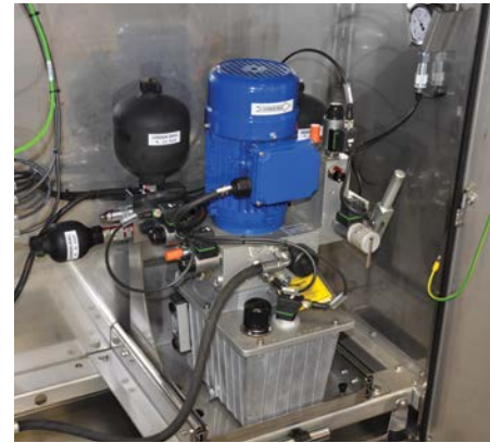
All Svendborg power units are designed and manufactured in-house to ensure compatibility with other Svendborg braking system components. Units are equipped to monitor oil level and temperature, motor and pump function, and system pressure.
