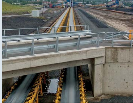
A 900 m (.55 mile) long overland conveyor, powered by three 500kW drives, installed at a large coal mine in Tusimice, Czech Republic.
