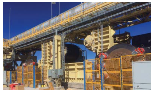
The entire four-flight, direct drive OGP1 conveyor system spans 10,632 m (6.6 miles) in length with the largest section being 3,942 m (2.4 miles) long.
