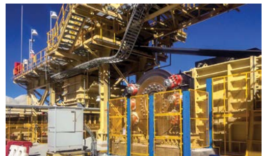
Groupings of six Model BSFB 650 spring-applied, hydraulically-released, dual-spring caliper brakes, acting on 2.7 m (8.8 ft.) diameter steel brake discs, serve as on/off holding brakes at the head of the various OGP1 conveyor sections.
