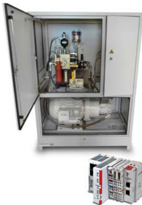
Pairs of SOBO® controllers and SOBO® hydraulic power units were installed on the OLAP conveyors. All Svendborg Brake power units are designed and manufactured in-house to ensure compatibility with other Svendborg braking system components. Units are equipped to monitor oil level and temperature, motor and pump function, and system pressure.
