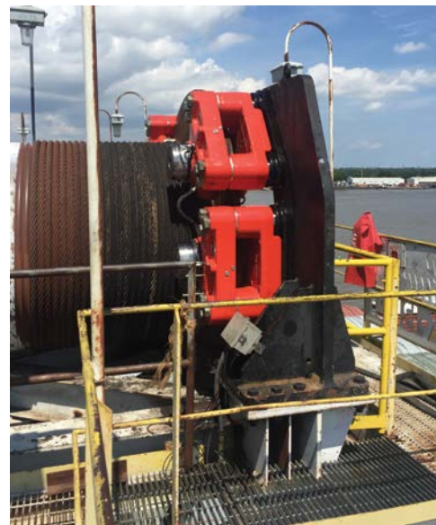
The braking upgrade allowed the use of the existing brake mounting pedestals saving an estimated $60,000 compared with the costs of completely replacing the system.
