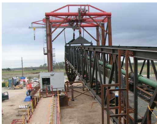
After fabrication and testing, the Marlin mining dredge was disassembled and loaded onto 23 tractor trailers for transport to the Florida "pond" where it will operate until the middle of the 21st century.
