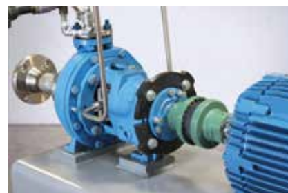
A size 7 TB Woods Sure-Flex® Plus coupling was able to be installed instead of a larger size 8 coupling on this small Group 1 Summit/GPM ANSI pump unit. By utilizing the smaller coupling, the overall package length was reduced allowing for a smaller baseplate footprint.
