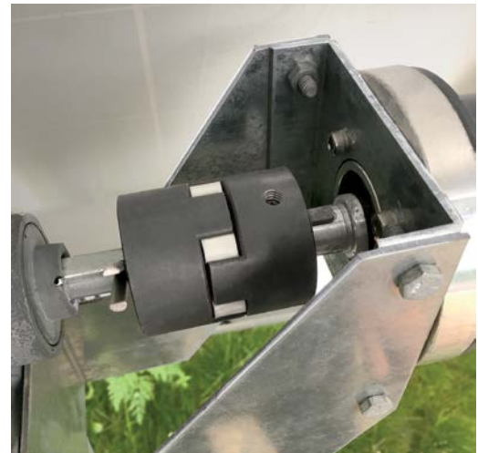
Reliable TB Wood’s L-Jaw couplings connect the drive motor to the driveshaft at the end of each row of PV modules.
