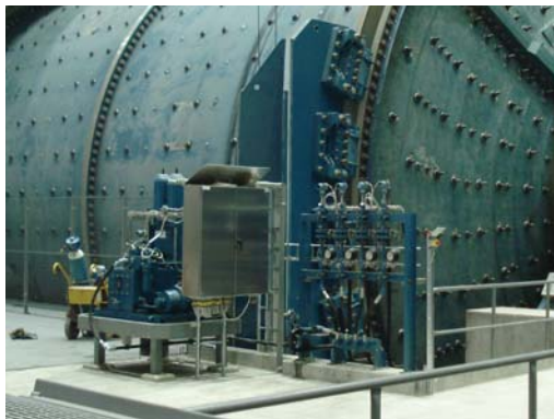
Twiflex Ltd. supplied eight VMS-DP brake calipers (with pedestals) plus a hydraulic power pack for each of the two primary mills.
