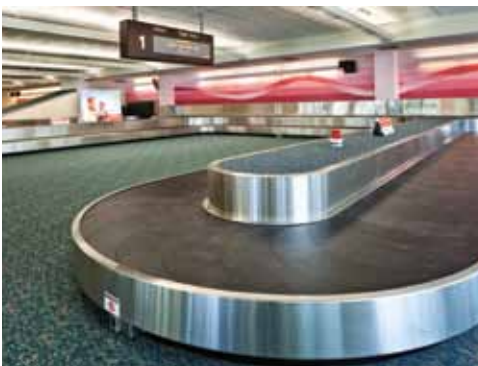
Thirteen new Siemens 300C Flat Plate baggage carousels installed at the Orlando International Airport feature unique distributed drive technology.
